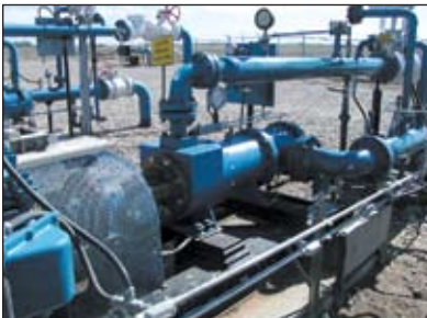
L3 re-engineered pumps replaced 3-screw pumps in crude oil charge application
