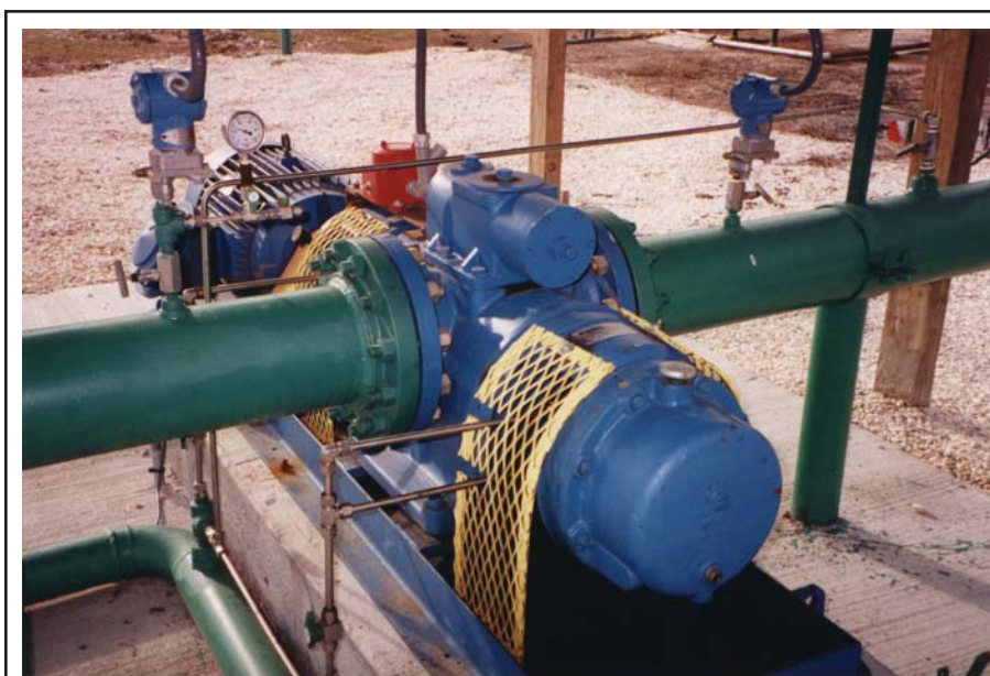
A multiphase pump was installed in the Humble Field north of Houston in 1998 to produce to a facility three miles to the south. The field was already more than 60 years old, and was barely flowing from beam-pumped wells. Today, the field is still in operation, with the multiphase pump continuing to extend the life of the mature property by boosting the pressure to reach the process facility while lowering the production manifold pressure.
