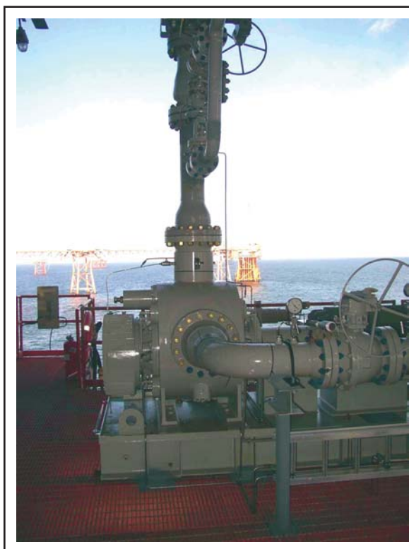
In a Gulf of Mexico field that had separate single-phase flowlines for oil and gas, a multiphase pump was installed after one of the lines failed, allowing McMoRan to begin transporting produced gas and liquids through the same line and avoiding the cost of replacing the second line. Courtesy of Texas A&M Multiphase Research Group.
